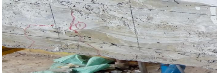
Fig 3.5 First Crack of GFRc Beam
