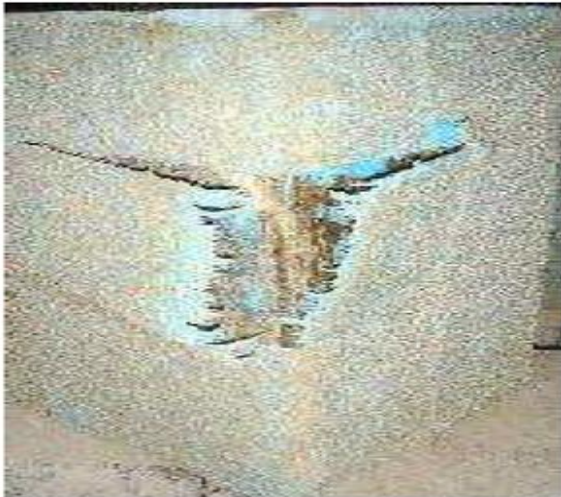
FIG No.3 GFRP WRAPPED SQUARE COLUMN WITH SHARP EDGES FAILURE OF FIBRE AT CORNER DUE TO STRESS CONCENTRATION
