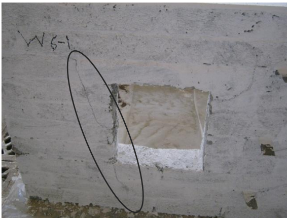
Figure (6): The crack pattern for tested wall specimen before rehabilitation
