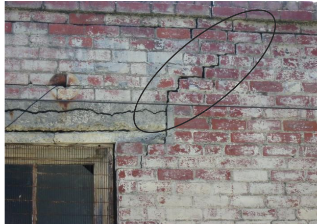
Figure (1): The cracking through the masonry developed primarily along the mortar joints in a diagonal stepping pattern at filed.
