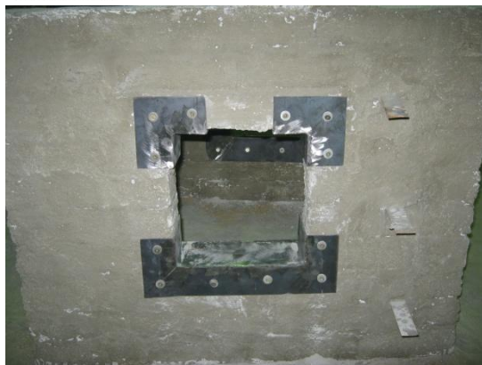
Figure (10): Details of the used rehabilitation technique using (2x60mm) L&U-shaped steel plate inside opening corners welded with U & L-shaped steel plate.
