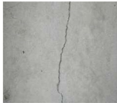
Fig. 12 Crack in Bacillus Subtilis sample after allowing for Self-healing
