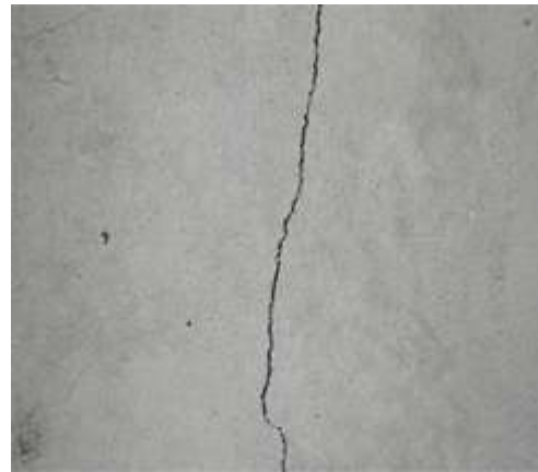
Fig. 11 Crack in Bacillus Subtilis Sample after 28 days of Curing
