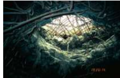
Fig. 1 The hole in Amiriyah Shelter's roof due to the U.S. aerial attack [3]
