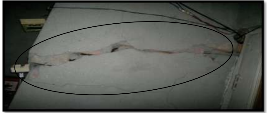
Stage II of Earthquake. Damage[1]
