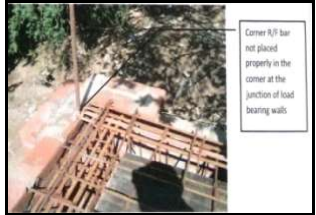
FIG D Misplaced vertical bar at the corner
