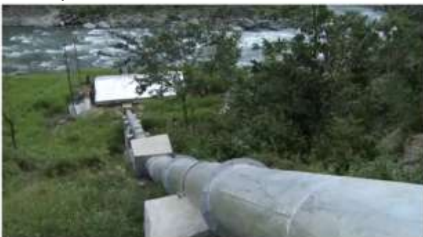
Fig 2. Nepal Micro Hydro Installation
