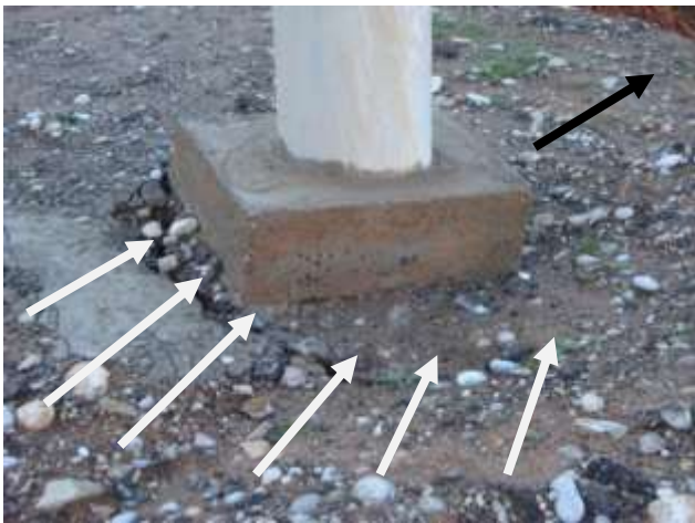
Fig. 4: The development of a crack at the foundation of electricity post due to progressive failure.
