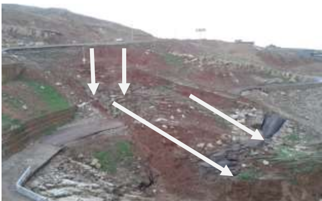
Fig. 5: A view of the failure and the damaged lower road (white arrows).
