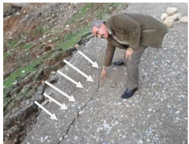
Fig. 3: The Start of crack development on edge of paved road due to progressive failure.
