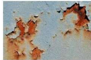
Fig 1: Example of a corroded metal surface.
