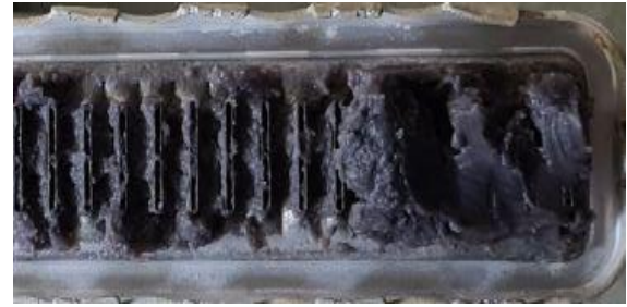
Fig. 11. Fragment of the radiator tube sheet in the area of the inlet pipe
