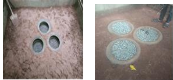
Fig 7: Model 3 foundation mounting, (a) Installation of tires into geogrid-mounted soil, (b) Finished installation of foundation model 3
