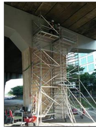
Fig. 4 Experimental AE installation under bridge
