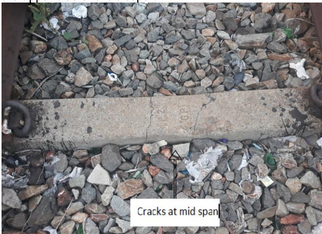
Figure 6 - Cracks of concrete sleeper
