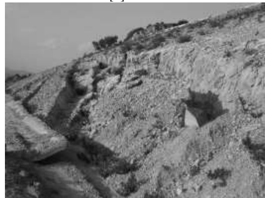
Fig 1 : Unhooking of materials from an excavation slope (Tetouan–Fnideq highway section)
