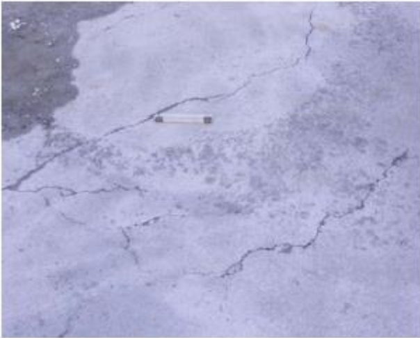
Fig 4: Plastic shrinkage cracks appearing on the concrete surface a few hours after placement [16].
