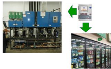
Fig. 3. Refrigeration Rack Controller controlling the store's refrigeration system to preserve the foods in the storage area.
