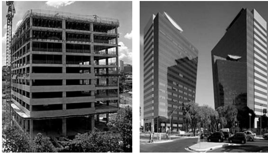
Figure 2: (a) Assembly of facade panels during the construction of Rochaverá Corporate Towers (b) Towers A and B of the building, completed in 2008 Source: [5]
