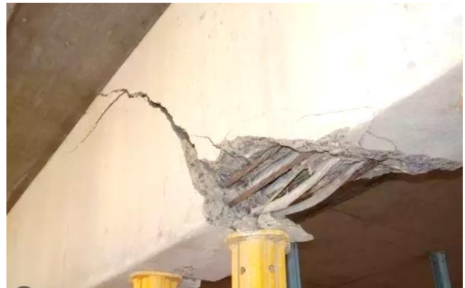
Fig. 4 Cracks on concrete structure
