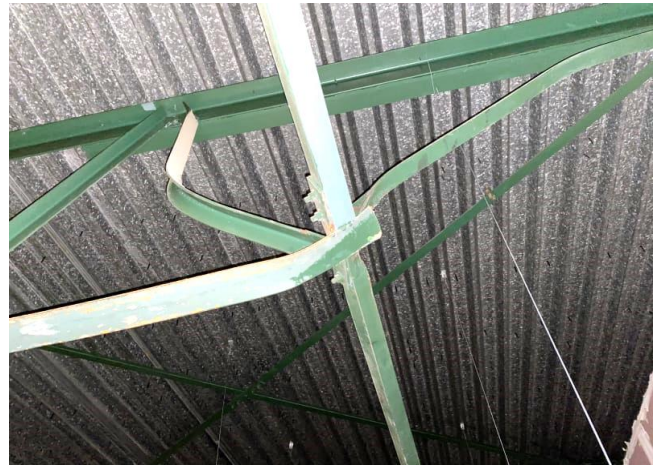
Fig. 3 Steel truss failure [5]
