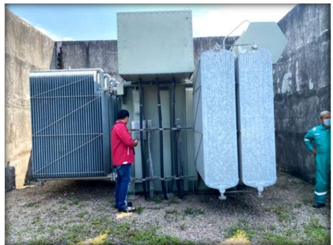
Fig. 2 Transformer 66 kV, 470 V at MMHE.
