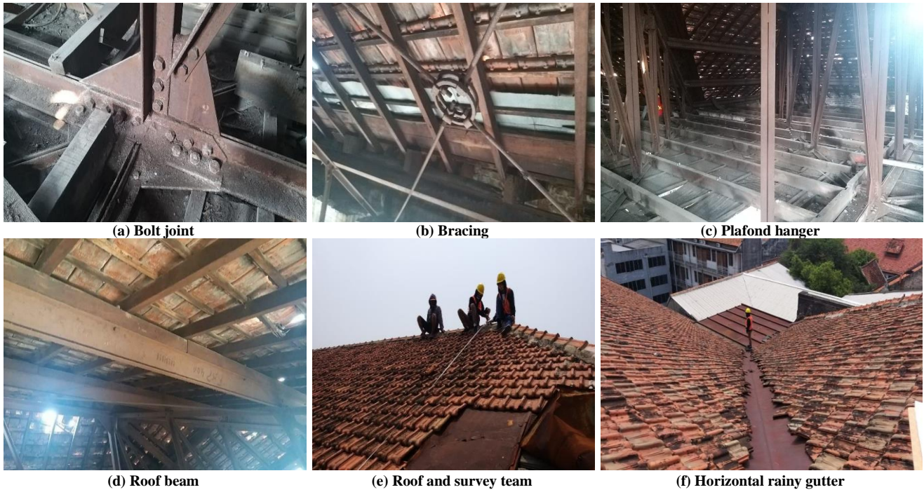
Fig. 11 (a), (b), (c), (d), (e), (f), (g) Existing detail roof structure and roof
